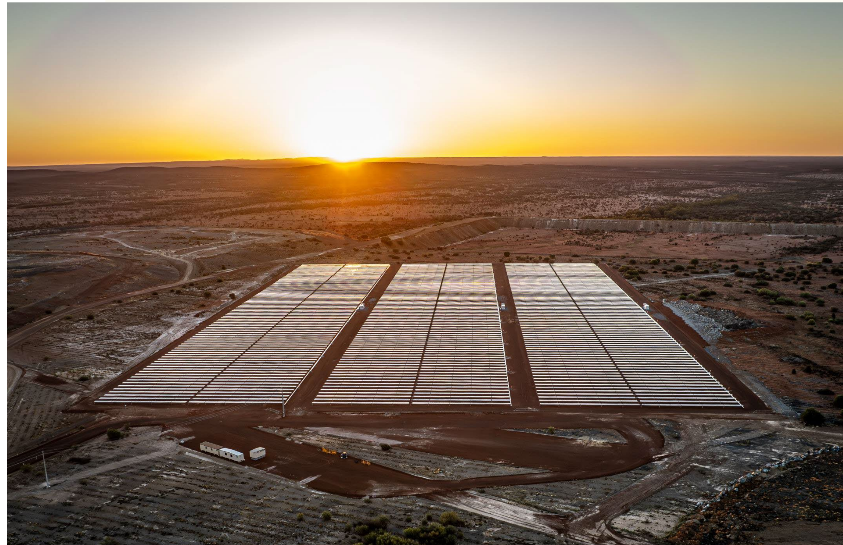
Bluebird solar farm commissioned in Q2 FY24
