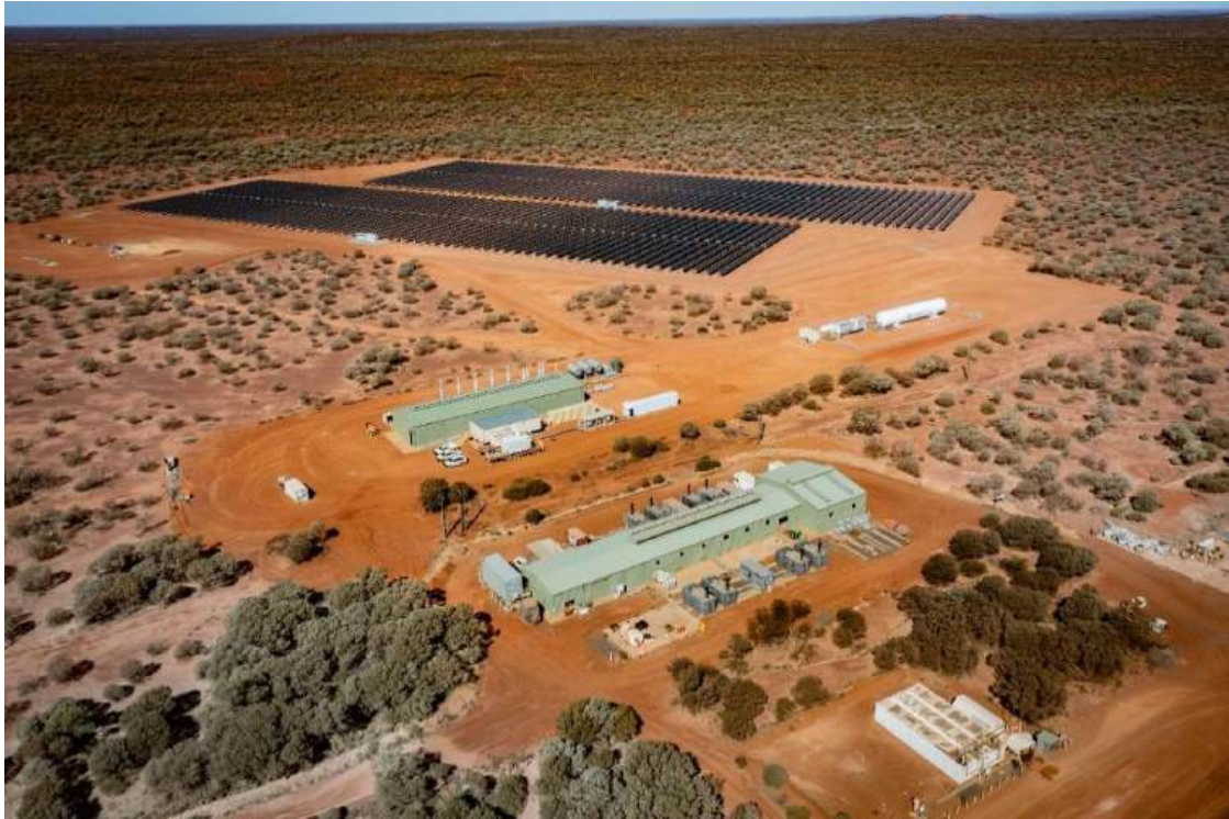
Figure 18-1 Tuckabianna solar farm and hybrid power generation facility. Source: Westgold.
