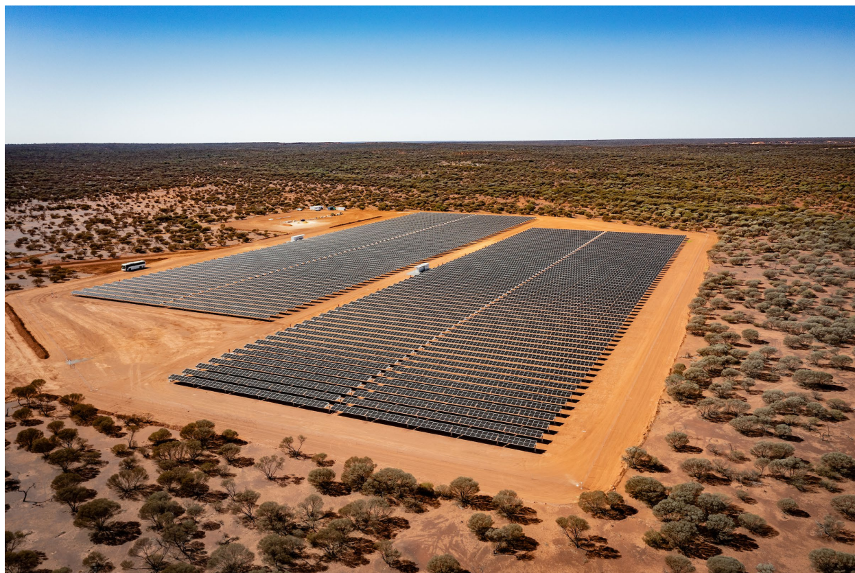
Figure 2 - 6MW solar farm at Tuckabianna
