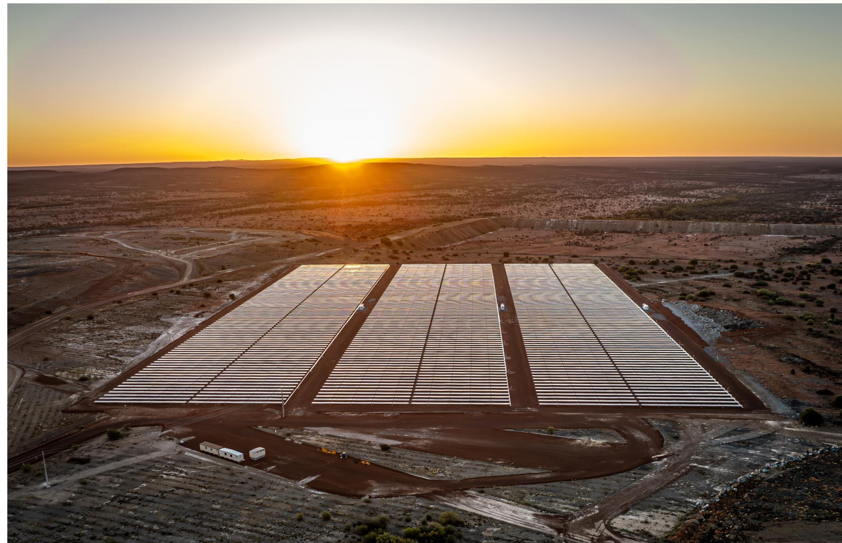
Bluebird solar farm commissioned in Q2 FY24
