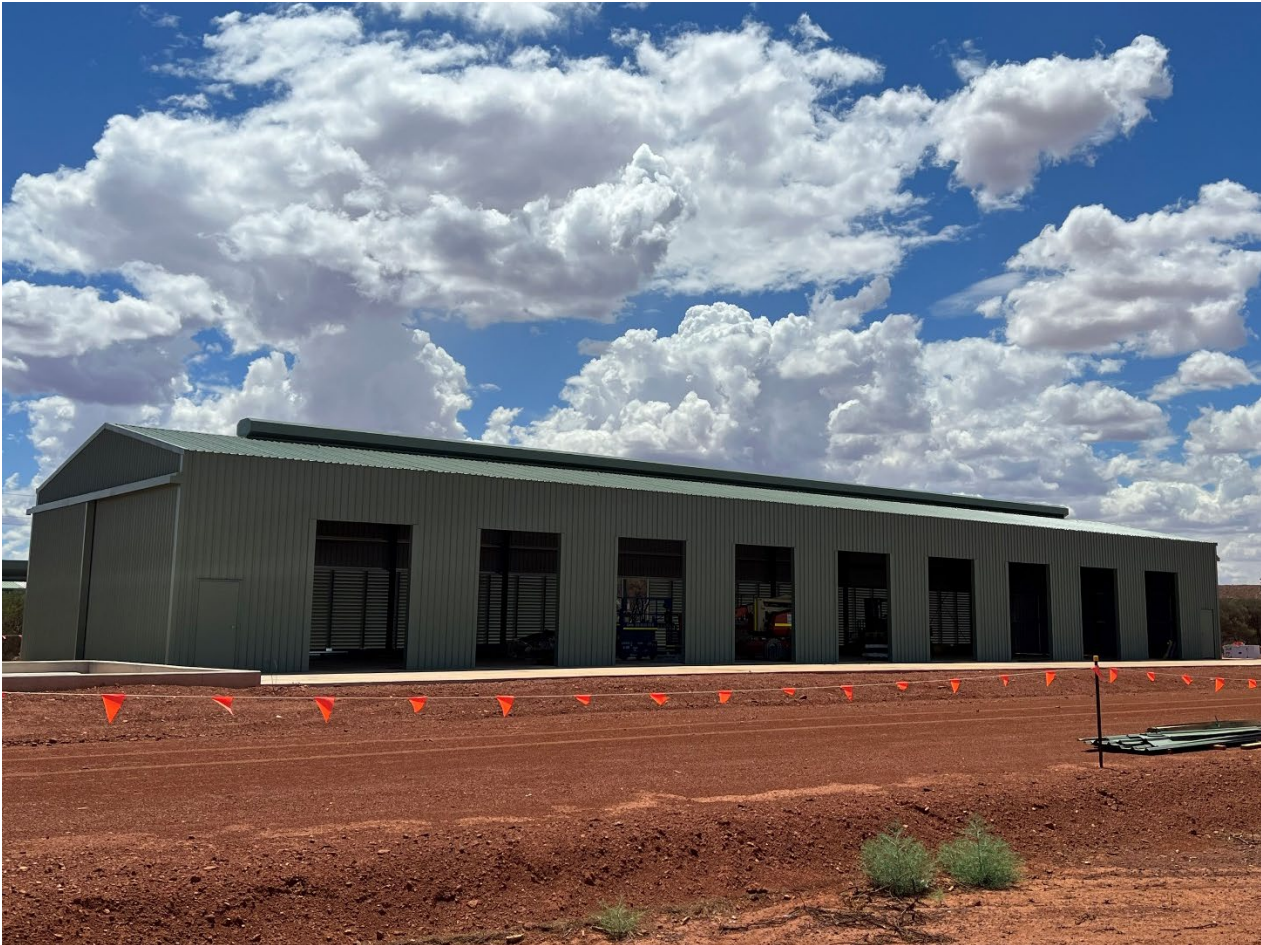
Figure 1 – New Gas Fired Power Station Enclosure under Construction at Tuckabianna Processing Hub
