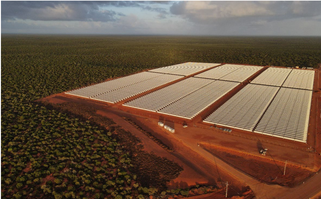
Figure 1: Renewable Energy – typical solar farm installation built by Pacific Energy at another operation in Western Australia
