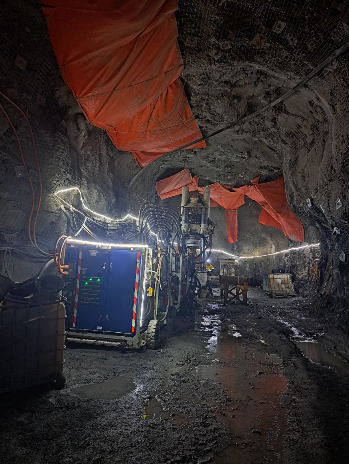
Figure 5 - Long-term ventilation infrastructure under development.
